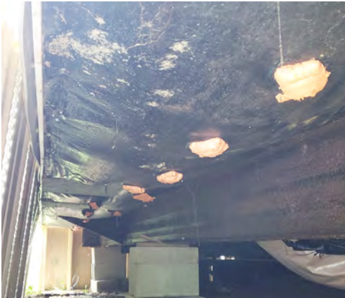
SPF belly patch: Installers use SPF to patch access holes in a mobile-home belly after blowing insulation.
