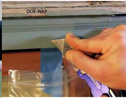
Cut through all the layers of paint. Also install a bag beneath the cut to catch paint fragments.
