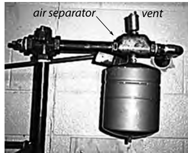
Expansion tank, air separator, and Vent: Preventing excessive pressure and eliminating air from the systems are important for hydronic distribution systems.
