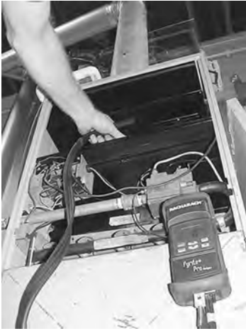
70+ Furnace: Sample flue gases within the draft diverter inside each exhaust port.
