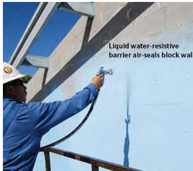
Liquid water-resistant barrier: This retrofit serves two purposes: water proofing and air sealing.
