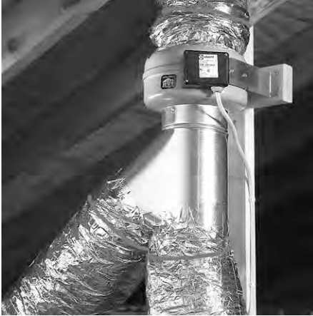
In-line fan in attic: A Y exhausts airflow from two bathrooms for both local exhaust and whole-building ventilation.
