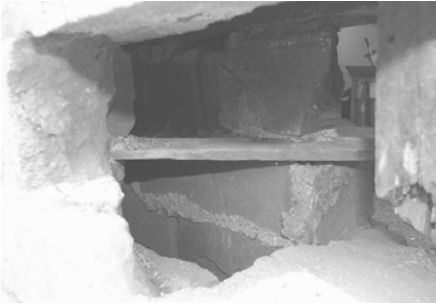
Cavity brick wall: Two separate single brick walls are held together by wood lath embedded in the mortar joint.
